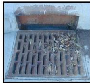
Photograph 8-6. Denver No. 16 Combination Inlet in need of maintenance (UDFCD Volume 1)
