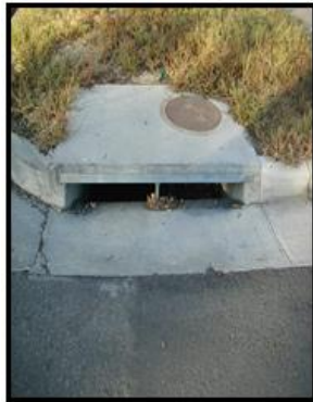
Photograph 8-4. Denver No. 14 Curb Opening Inlet (UDFCD Volume 1)
